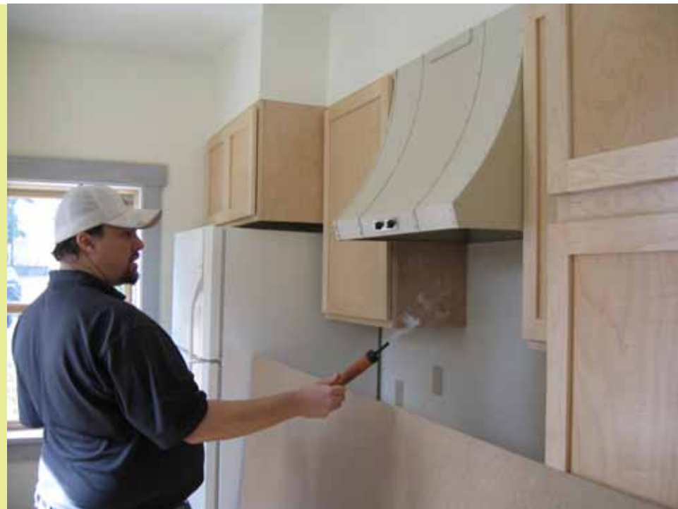
Testing exhaust fans for flow helps confirm minimal ventilation rates are being met, promoting healthy indoor air quality and reducing the likelihood of moisture damage.
