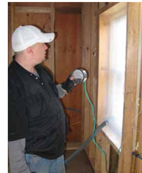
Professional envelope inspections can identify air leaks and potential future moisture problems easily overlooked in a visual inspection.
